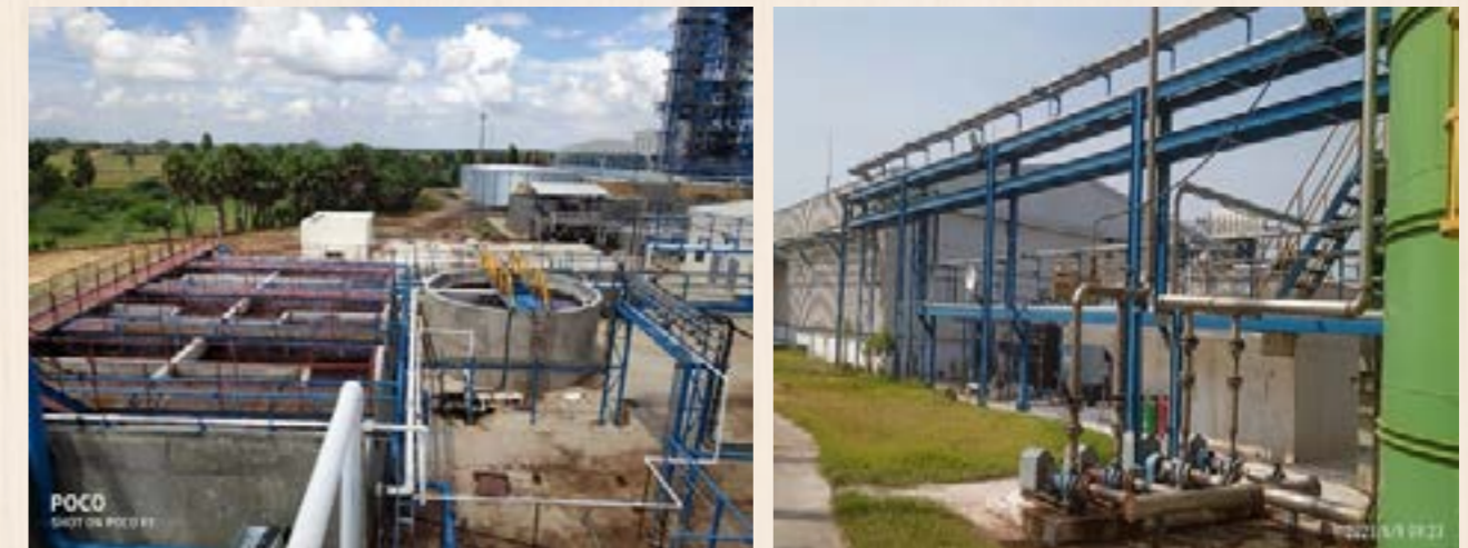
Installed ETP STP
